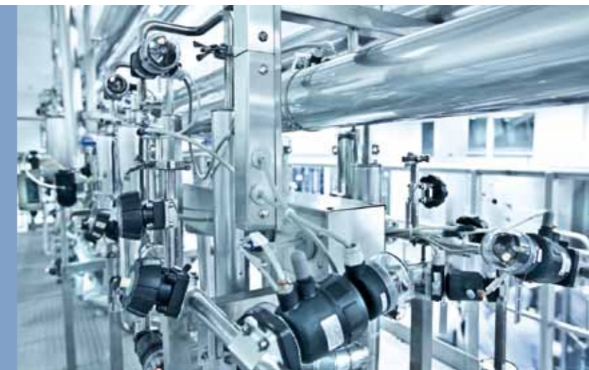
Fittings installation in the cleanroom of the new LIFE Nutrition plant at B. Braun in Melsungen
